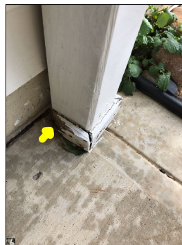
Wood rot damage along the column.
