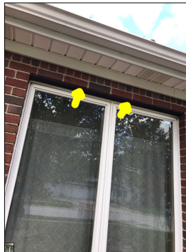
Rust and corrosion along the header. This is considered a defect.
