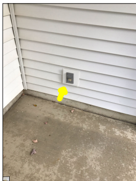
The weather protection cover is missing.
