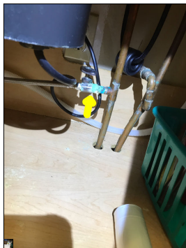
Rust/corrosion along the plumbing pipes.
