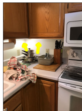
The light is noisy during operation. This is considered a defect.
