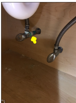
Rust/corrosion along the plumbing pipes.
