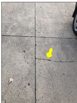
Cracks and deterioration along the driveway.
