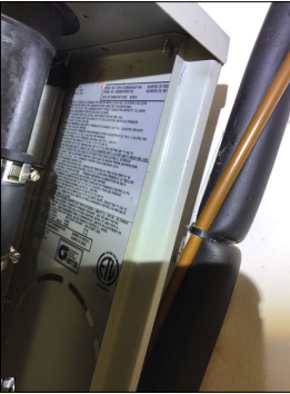
Furnace data plate.
