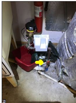
Main water shut off valve.
