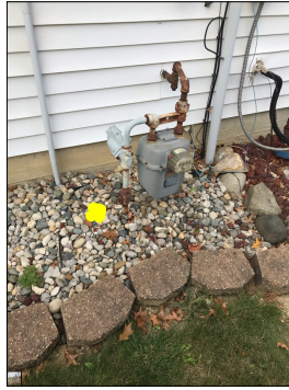
Main fuel shut off valve.
