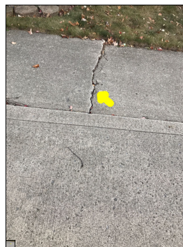
Cracks and deterioration along the driveway.
