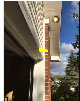
Dents along the siding.
