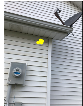
Gaps along the siding.
