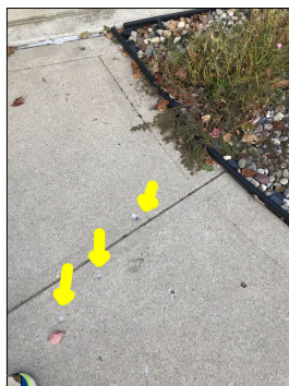
Pitting along the service walks.
