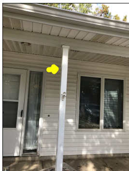
The column is loose.
