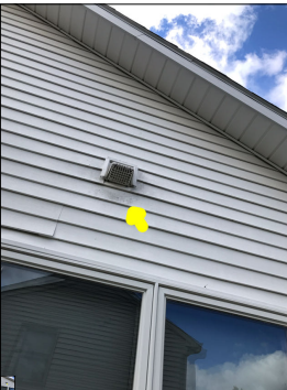
Discoloration along the siding.
