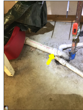
The garage sink unconventionally drains into the floor drain. This is considered abnormal and amateur craftsmanship. The sink should drain into the main drain pipes.
