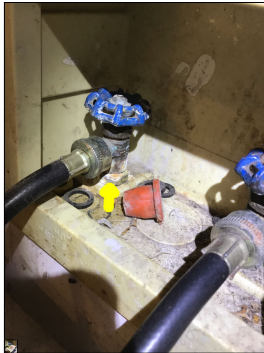
Corrosion along the water lines. This is located in the garage.
