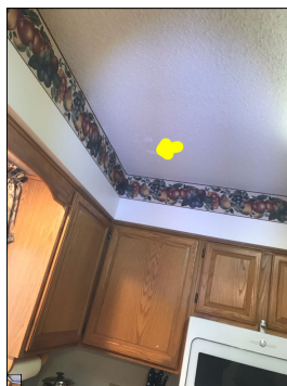
Discoloration along the ceiling.
