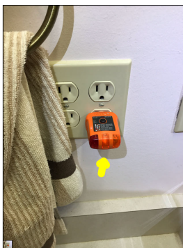
Open ground receptacles
