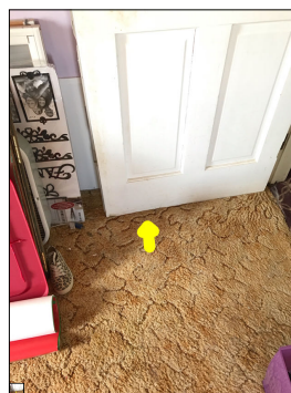
The door drags the floor during operation.
