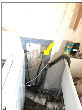
Rust/corrosion along the washer hook up lines.
