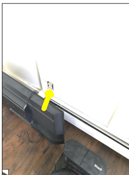
Missing receptacle covers.
