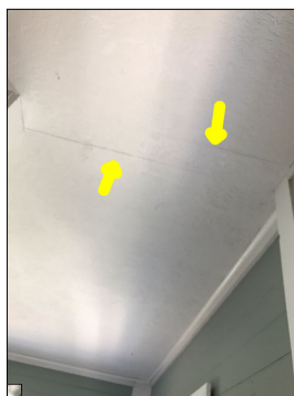
Cracks along the ceiling.
