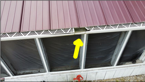
Missing section of gutter guards.
