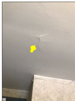
Cracks along the ceiling.
