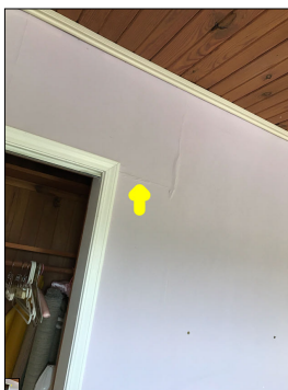
Cracks along the walls.
