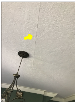
Cracks along the ceiling.
