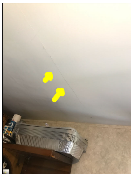
Cracks along the ceiling.
