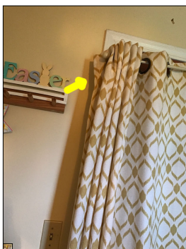
The door does not properly close.
