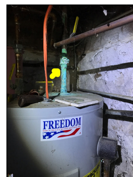
Corrosion along the water supply lines.
