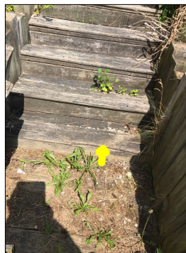
Deterioration along the service walks.
