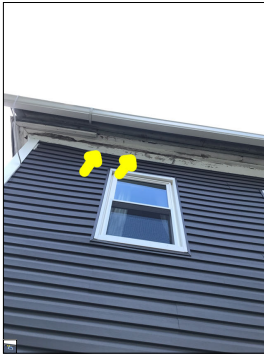
Flaking and peeling along the siding.
