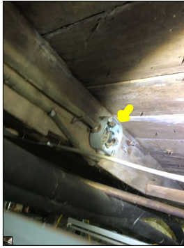
Open junction boxes.
