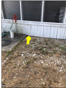
Wood rot damage.
