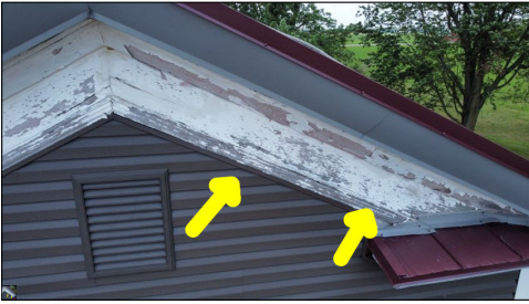
Flaking and peeling along the siding.
