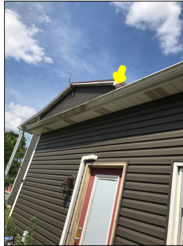
Loose gutter spikes.
