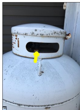
Main fuel shut off valve.
