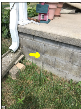
Cracks and deterioration along the porch.
