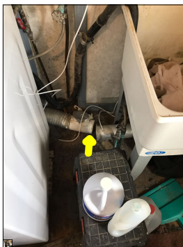
The ductwork is disconnected.
