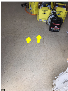
Cracks and deterioration along the patio.
