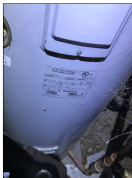
Water heater data plate.
