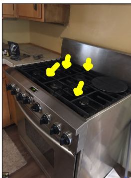
Inoperable burners. The burners do not ignite.
