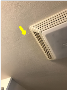
Cracks along the ceiling.
