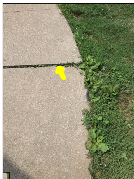
Uneven surfaces along the service walks.
