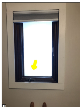
Aged and inoperable window.
