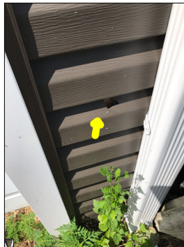
Holes along the siding.
