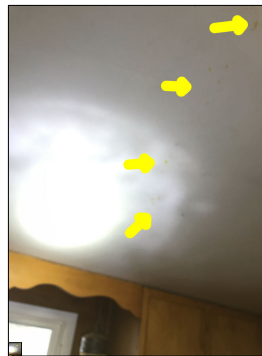
Discoloration along the ceiling.
