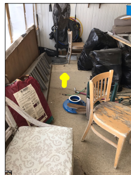
Cracks and deterioration along the patio.
