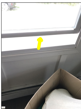
Missing window screens.
