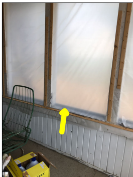
Unconventional plastic along the windows. This is considered abnormal.
