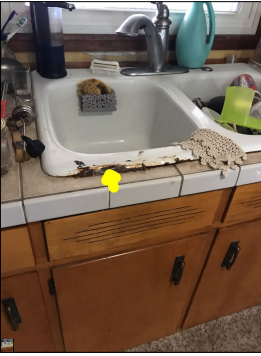
Rust and corrosion along the sink.
