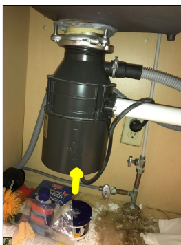
The garbage disposal is inoperable.
