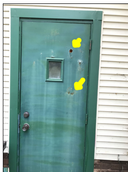
Rust and corrosion along the door.
