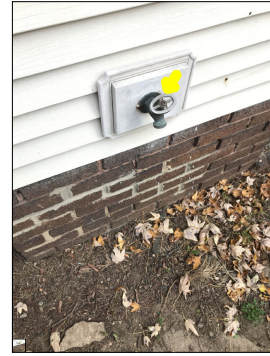
Inoperable hose bib.
