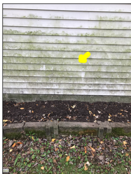
Discoloration along the siding.
