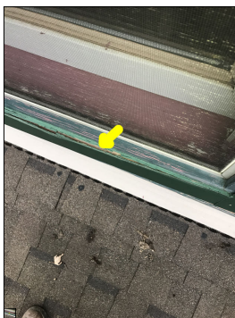
Gaps along the siding.
