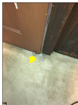
Torn weatherstrip along the door.
