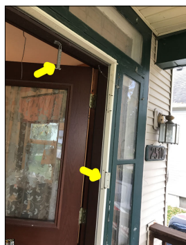
Missing storm door.
