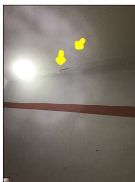
Cracks along the ceiling.
