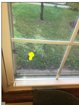
Holes along the window screen.
