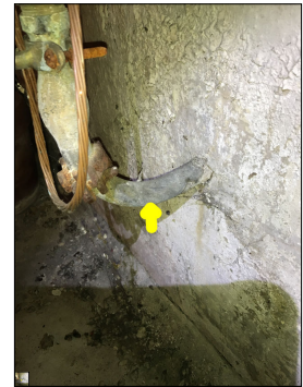
Lead water supply pipes. Lead pipes are a potential safety hazard. Recommend upgrading from lead pipes to modern day water supply pipes, such as PEX or copper.
