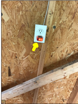
Non GFCI protected receptacles.
