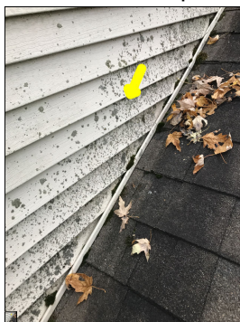
Discoloration along the siding.
