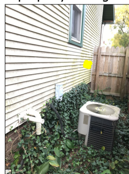
Discoloration along the siding.
