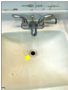
Missing drain stopper.
