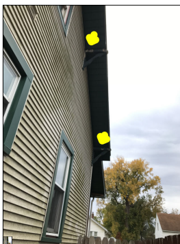
Flaking and peeling along the siding.
