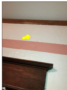
Cracks along the walls.
