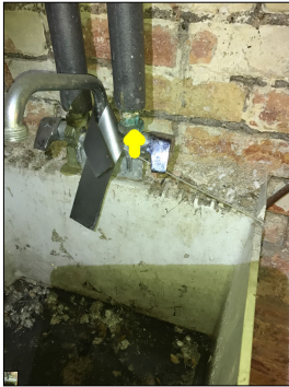
Rust and corrosion along the plumbing pipes.
