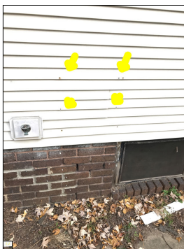
Holes along the siding.
