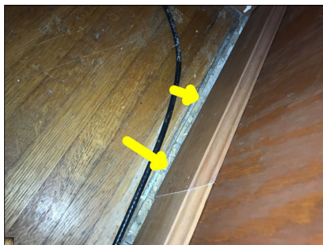
Gaps along the floor.
