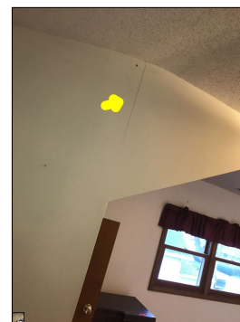
Cracks along the walls.
