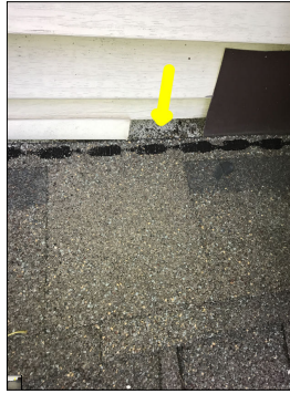
Unconventional flashing. Water can get underneath the shingles. This is a potential leak point area.
