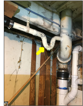
Unconventional running trap. This is considered abnormal and a defect. A running trap can catch debris and create blockage. Also, a running trap is difficult to clean due to restricted access.
