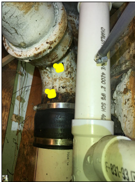
Rust and corrosion along the plumbing pipes.
