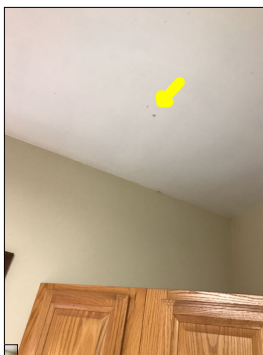
Discoloration along the ceiling.
