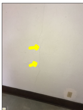
Cracks along the walls.
