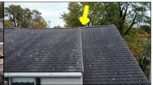
The ridge line is sagging. This is considered abnormal and a structural defect.
