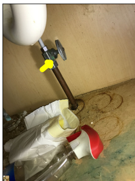
Rust/corrosion along the plumbing pipes.
