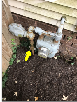
Main fuel shut off valve.
