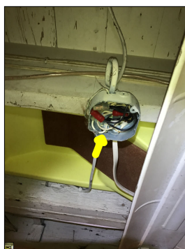
Open junction boxes.
