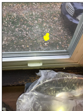
Holes along the window screen.
