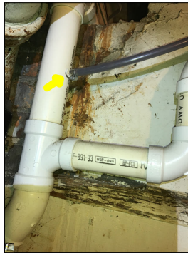
Unconventional condensation line routed into the drain pipe. The connection is improper. There needs to be a p trap below the connection point. The current connection can allow sewer gases into the house, thus creating a potential safety hazard.
