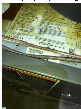
Furnace data plate.
