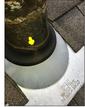
Torn flashing. This is a potential leak point. Water intrusion into the attic and house can cause property damage and mold growth.
