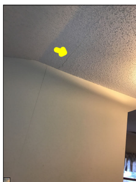
Cracks along the ceiling.
