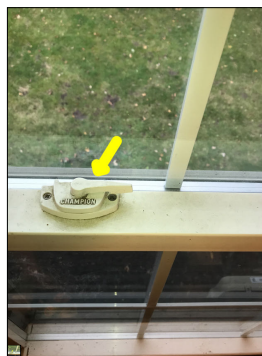
The window lock does not properly align with the latch keeper. This is considered a defect.
