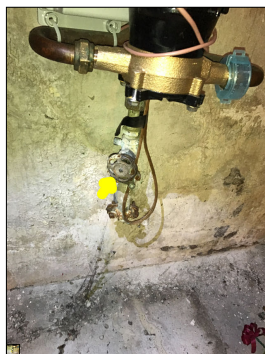
Main water shut off valve.
