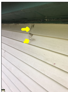
Unconventional application of caulk and repairs along the siding. This is considered abnormal and amateur craftsmanship.
