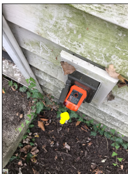
Non GFCI protected receptacles.
