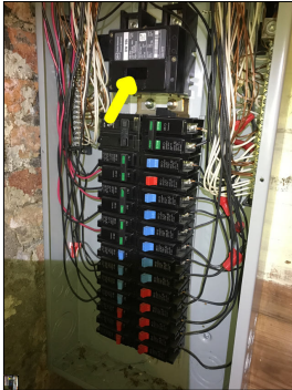
Main circuit breaker.
