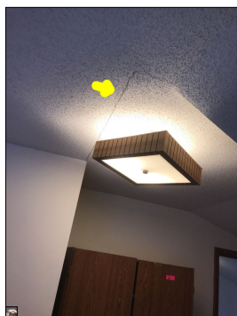
Cracks along the ceiling.
