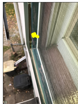
Gaps along the siding.
