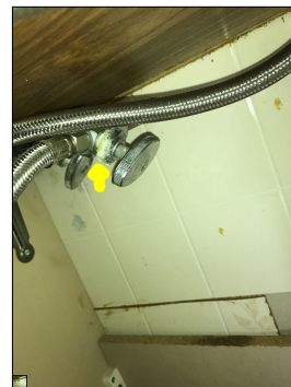
Rust/corrosion along the plumbing pipes.
