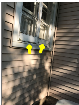
Flaking and peeling along the exterior.
