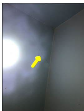
Cracks along the walls.
