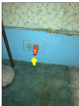
Non GFCI protected receptacles.
