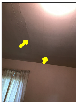
Cracks along the ceiling.
