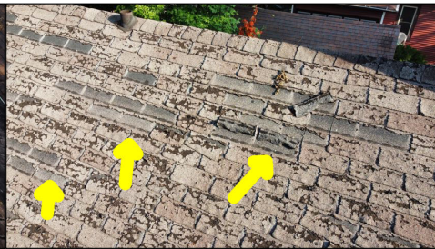
Damaged and deteriorated roof shingles.
