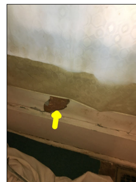
Flaking and peeling along the walls.
