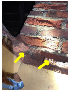
Deterioration and cracking along the brick.
