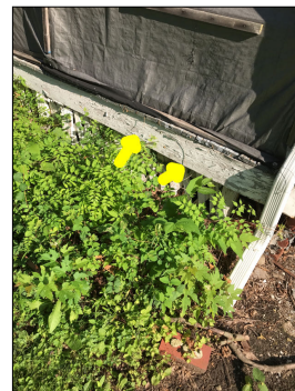
Flaking and peeling along the exterior.
