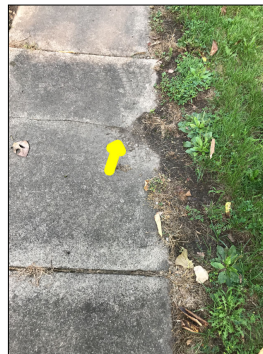
Cracks and deterioration along the service walks.
