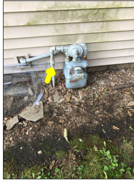
Main fuel shut off valve.
