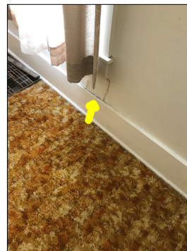
Cracks along the walls.
