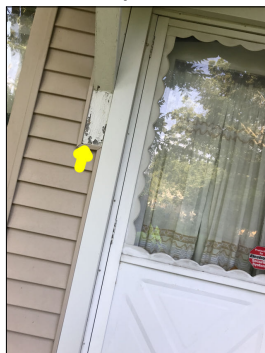
Flaking and peeling along the exterior.
