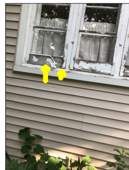
Flaking and peeling along the exterior.
