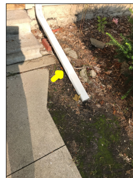
Dents along the gutter system.
