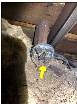
Exposed spliced wires. This is a potential safety hazard.
