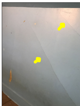
Cracks along the walls.
