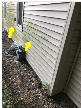
Discoloration along the siding.
