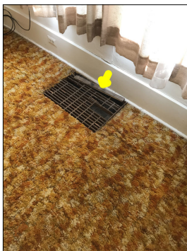
Damaged vent covers.
