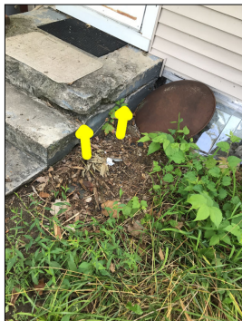
Cracks and deterioration along the service walks/steps.
