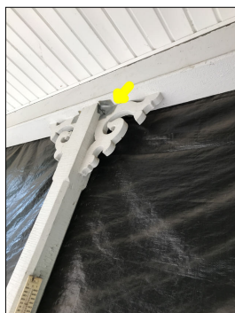
Unconventional tape along the porch.
