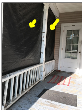
Unconventional tarp along the porch. This is considered abnormal.
