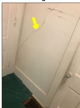
Cracks along the walls.
