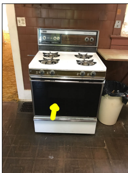
Aged range. The range is inoperable.
