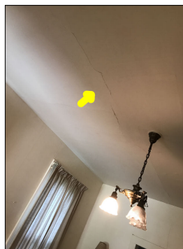
Cracks along the ceiling.
