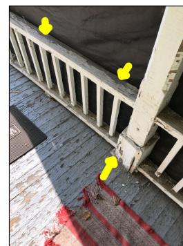
Flaking and peeling along the porch.
