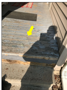
Flaking and peeling along the porch.
