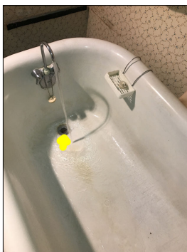
Missing original drain stopper.
