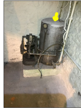
Aged pressure tank in the basement. The tank is not in service.
