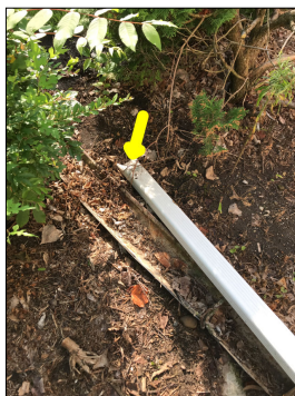
Smashed gutter extension.
