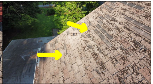
Damaged and deteriorated roof shingles.
