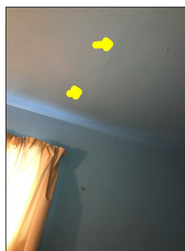
Cracks along the ceiling.
