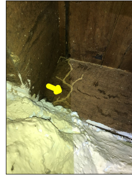
Signs of termite damage. Termites are a wood destroying insect and can cause property damage and structural damage.
