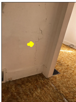
Cracks along the walls.
