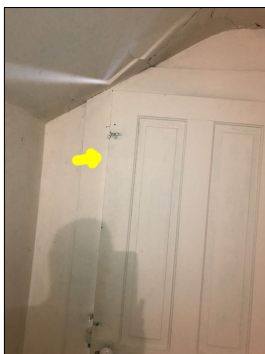
The door does not latch properly.
