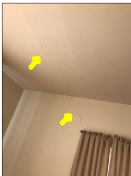
Cracks along the ceiling and walls.
