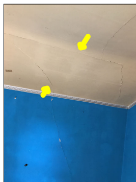
Cracks along the ceiling.
