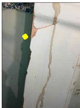
Flaking and peeling along the walls.
