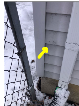
Holes along the siding.
