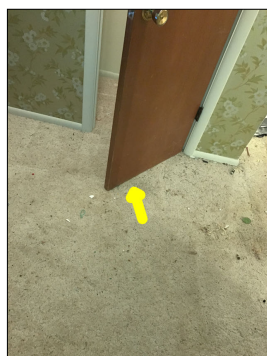
The door drags the floor during operation.
