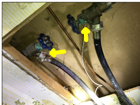
Rust/corrosion along the washer hook up lines.
