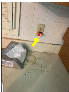
Non GFCI protected receptacles.
