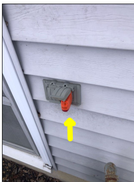
Non GFCI protected receptacles.
