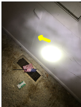
Cracks along the walls.
