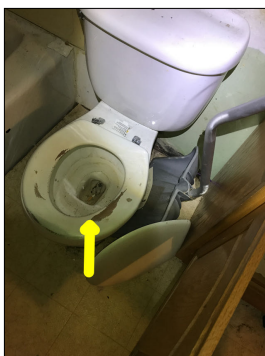
The toilet is inoperable.
