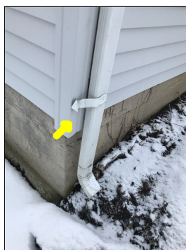
The downspout is loose.
