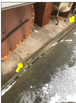
Cracks and deterioration along the floor.
