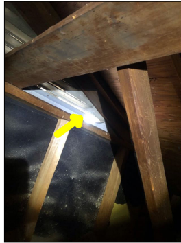
Damage/holes along the gable vent. A damaged gable vent can allow the intrusion of wildlife. Wildlife activity can cause property damage.
