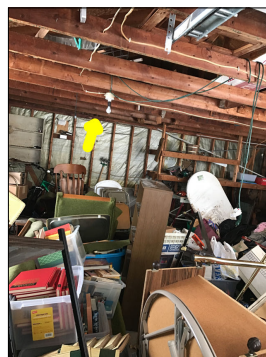
The light is inoperable.
