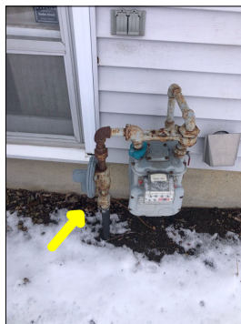
Main fuel shut off valve.
