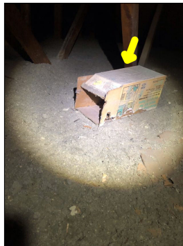
Debris within the attic.
