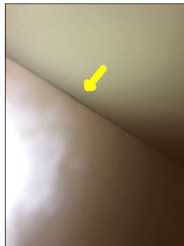
Cracks along the ceiling.
