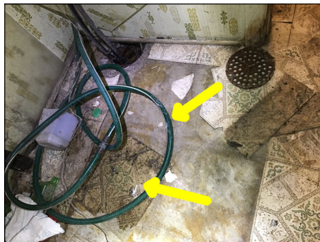
Moisture/water observed. This is considered a defect. An active or intermittent water source can cause mold growth and property damage.
