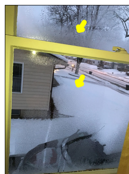
Condensation along the windows. This is considered a defect. An active or intermittent water source can cause mold growth and property damage.
