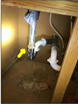
Rust/corrosion along the plumbing pipes.
