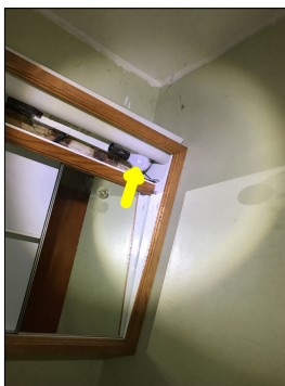
The light is inoperable.
