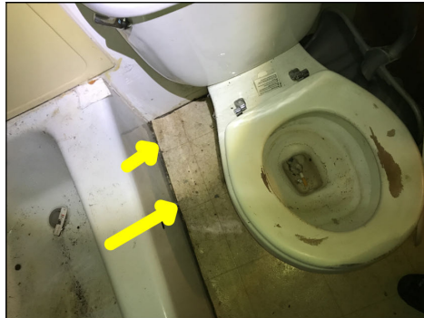
The flooring is loose.
