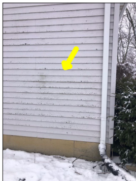
Discoloration along the siding.
