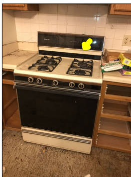
The range is inoperable.
