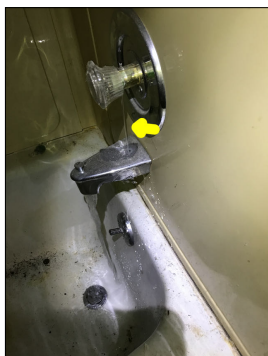
The faucet/handle leaks during operation.
