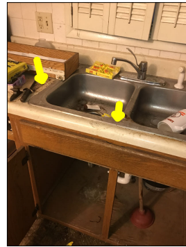
Excessive debris along the countertops.
